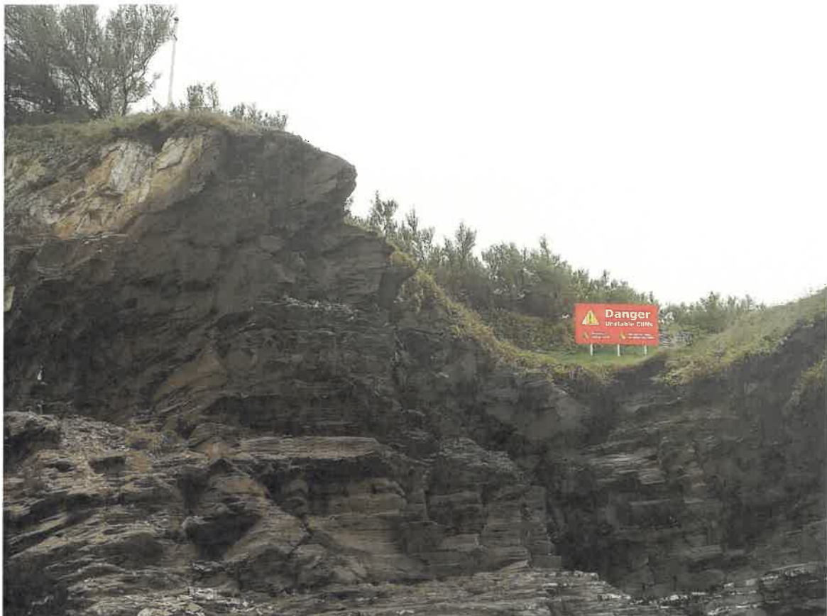
Picture above taken on the afternoon of the works by Council Facilities Officer. Shows the scaling section on the left hand side and give different perspective of the whole ledge/cliff area.
